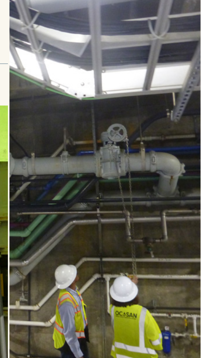
Troubleshooting to improve system operation and facility longevity.
