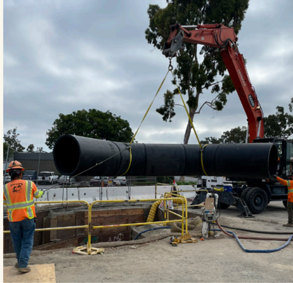
Installing an angled piece of pipeline on the Baker Force Main Rehabilitation, Project No. 7-65, in the City of Costa Mesa.
