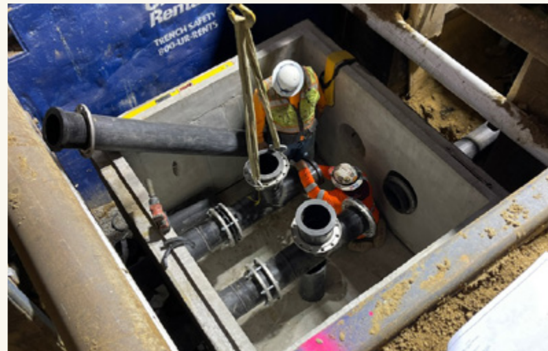
New dual force mains and access structure on the MacArthur Force Main Improvements, Project No. 7-68.
