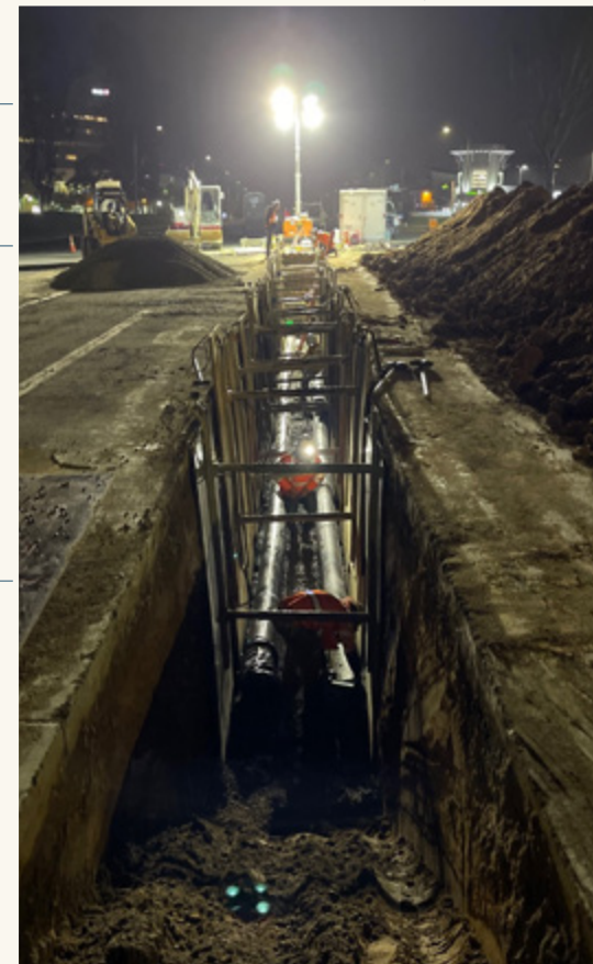
Most of the construction occurred during the nighttime hours to reduce impacts to the business community and traveling public on the MacArthur Force Main Improvements, Project No. 7-68, in the City of Newport Beach.
