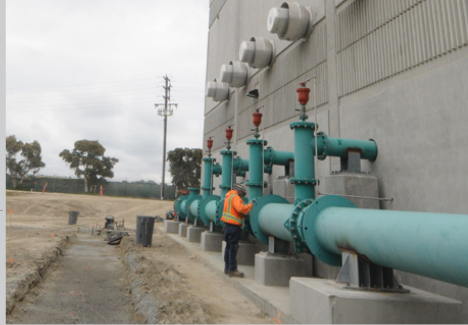
Fastening pieces of the plant water pump station discharge piping on the Outfall Low Flow Pump Station, Project No. J-117B.
