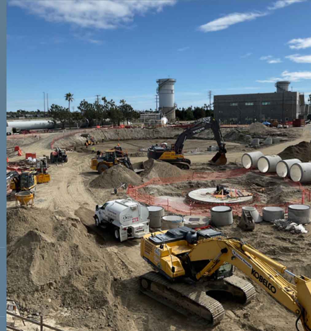
A-Side Clarifiers Replacement at Plant No. 2, Project No. P2-98A, in the City of Huntington Beach.
