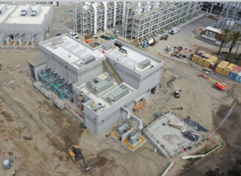
New Low Flow and Plant Water Pump Station as part of the Outfall Low Flow Pump Station, Project No. J-117B.
