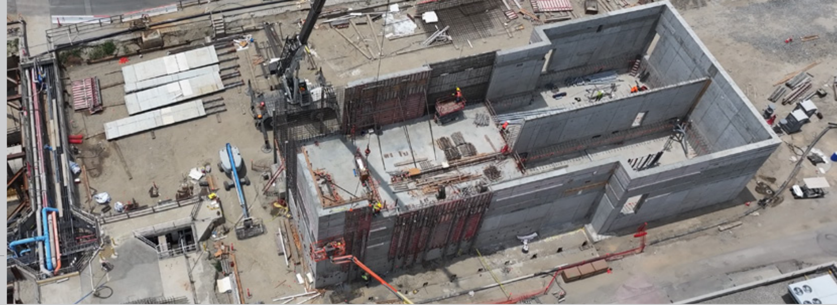
Construction of exterior concrete walls of a new electrical building for the A-Side Primary Clarifiers Replacement, Project No. P2-98A.
