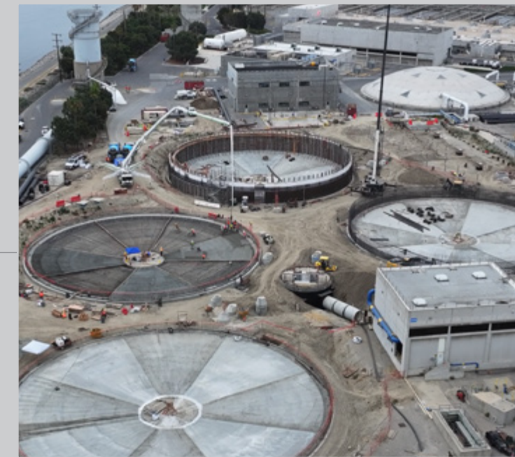
The A-Side Primary Clarifiers Replacement at Plant No. 2, Project No. P2-98A, will construct four new primary clarifiers.
